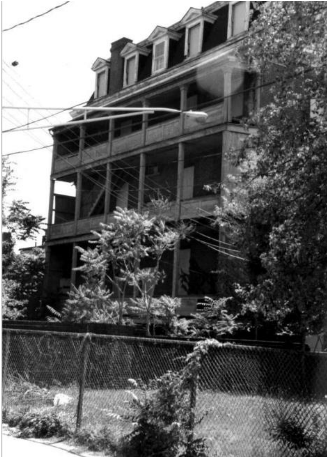
Image 17: The rear [east] elevation of the Home of the Friendless in June 2002 (Fred B. Shoken, "Home of the Friendless" National Register of Historic Places Nomination Form (Washington, DC: U.S. Department of the Interior, National Park Service, 2002))
