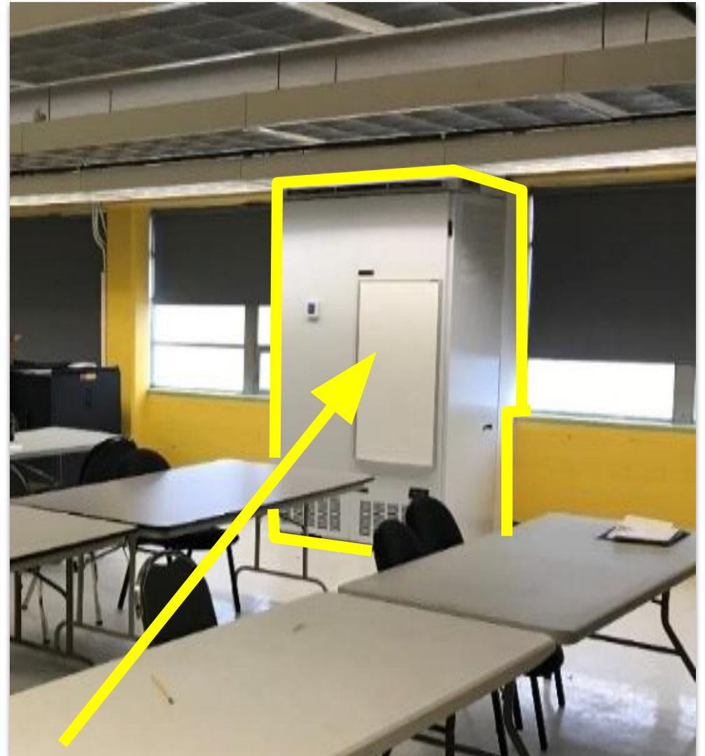
Vertical Package Unit (VPU) complete at Reginald F. Lewis
