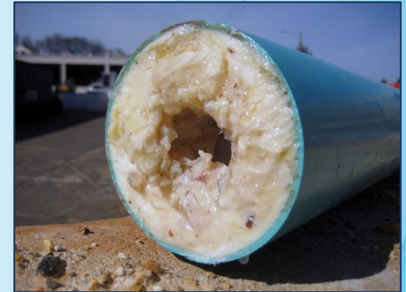
Fats, Oils and Grease (FOG)
