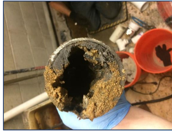
Debris, Rags, diapers, disposable wipes, etc
