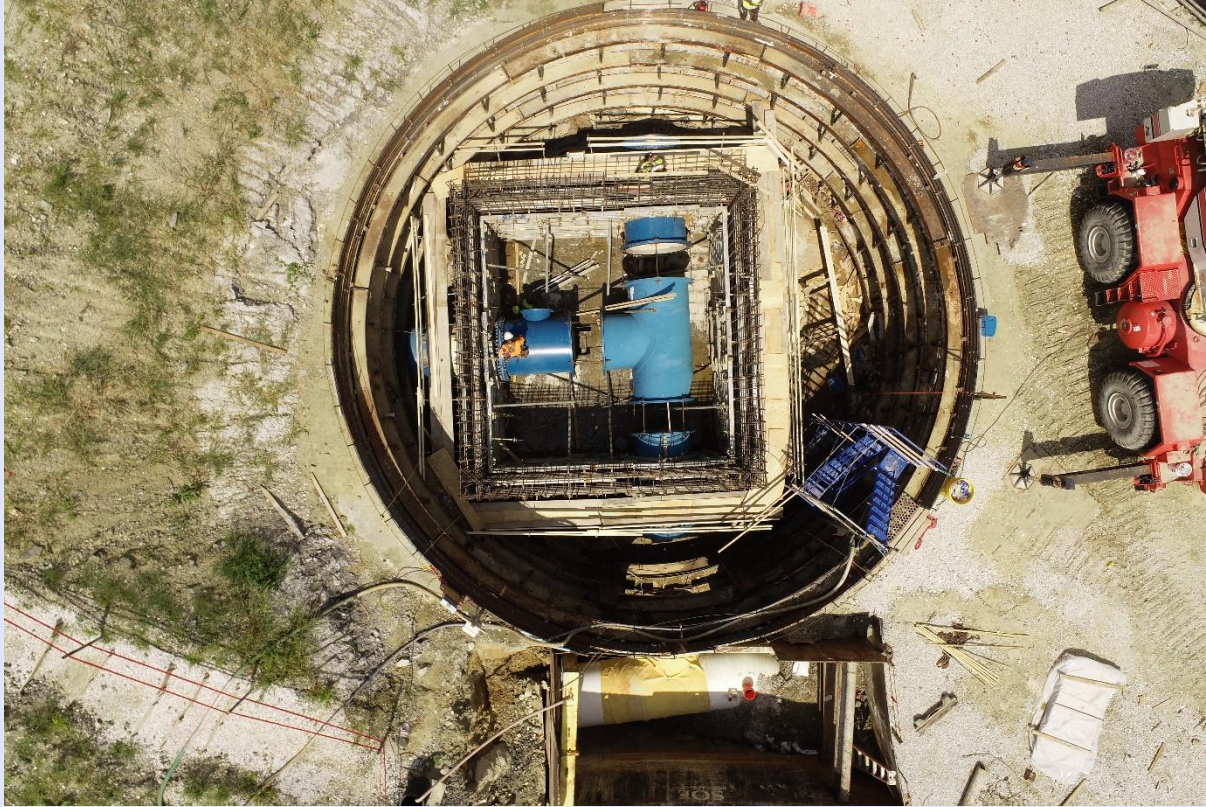
60 x 66" tee within B/F Vault – 8/10/2022
