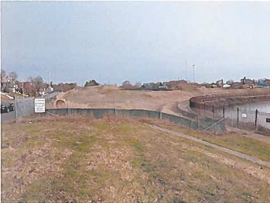
Photo 17: A view to the north along N. Hilton Street, with the construction work visible.
