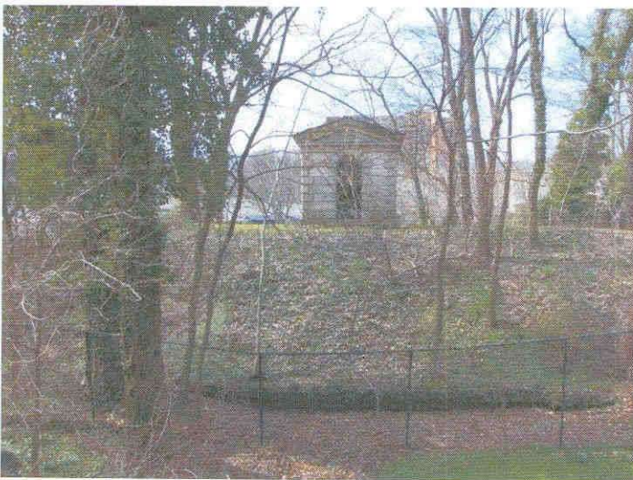
View from Falls Road of the Cross Keys Valve House, located on the embankment over the defunct conduit.
